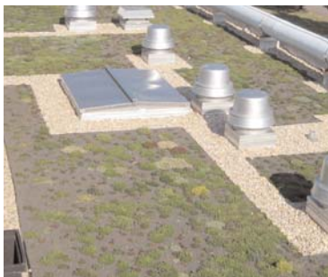
HRSD installed a green roof to filter stormwater and extend roof life.
